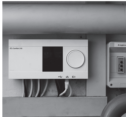
District Heating Controls
