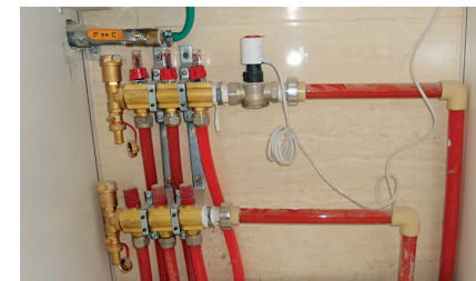
Danfoss manifold with RA-G valve and TWA-A actuator. This combination was installed in the smaller apartments to provide central temperature control via a CWD thermostat in the main living room. Individual room controls were installed in the larger apartments.
