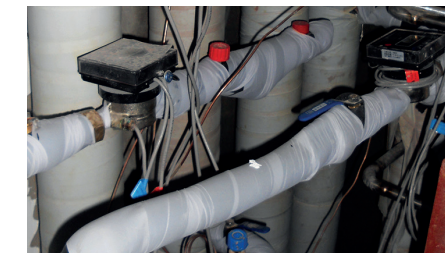
Danfoss ASV balancing valves and energy meters were installed in the technical room for each group of four apartments.
